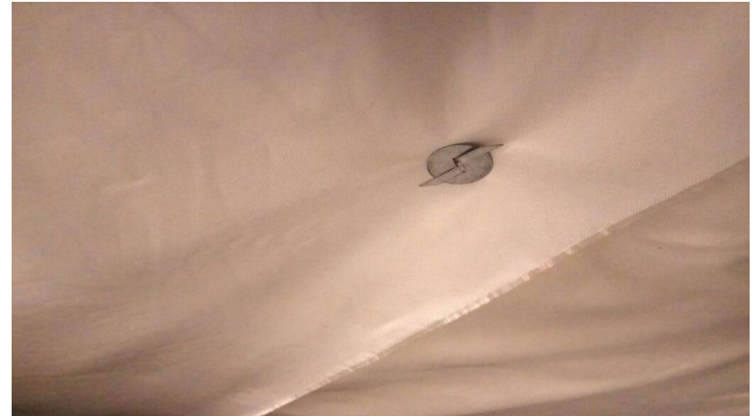
Washer on Tip of Insulation Anchor [Installed on Glass Cloth Surface]
